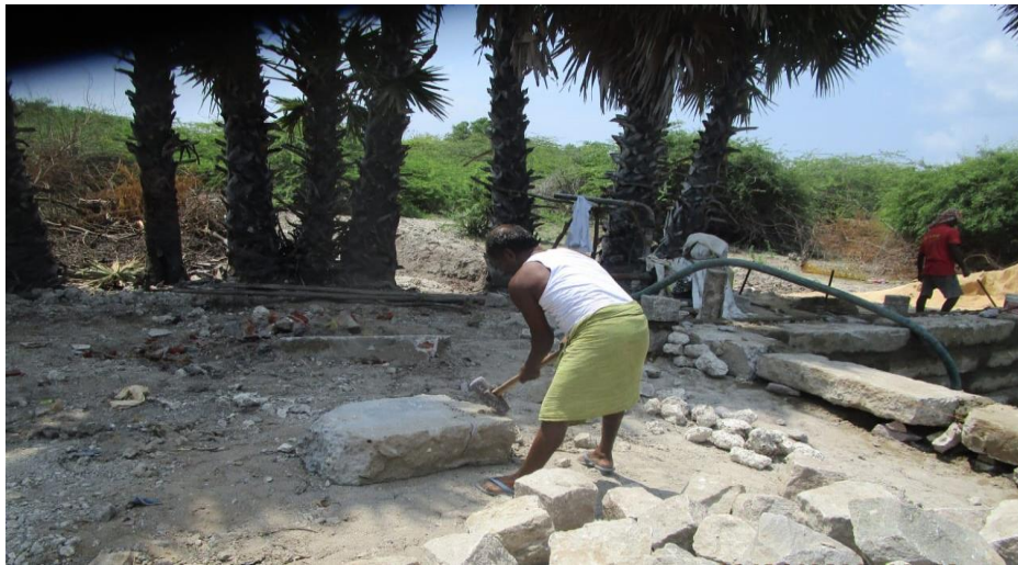
Recycle – Reuse - old stones are cut to size for the new construction
