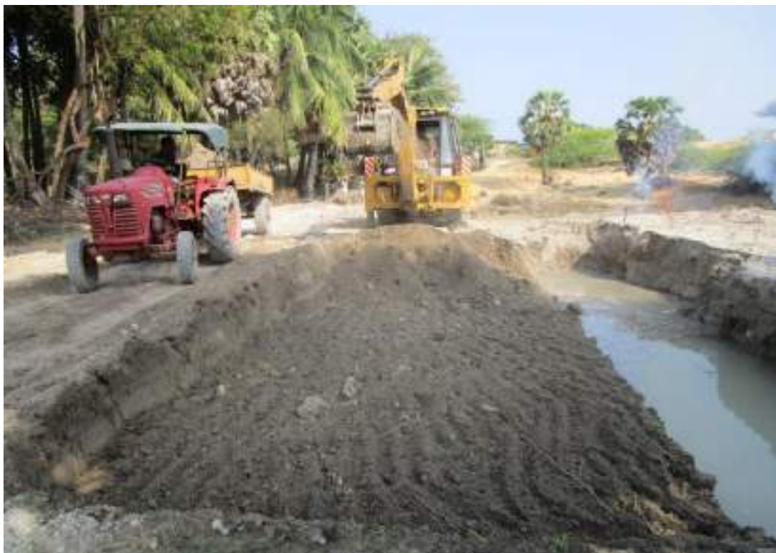
Basic Excavation work is on and the soil is carried away for laying the road
