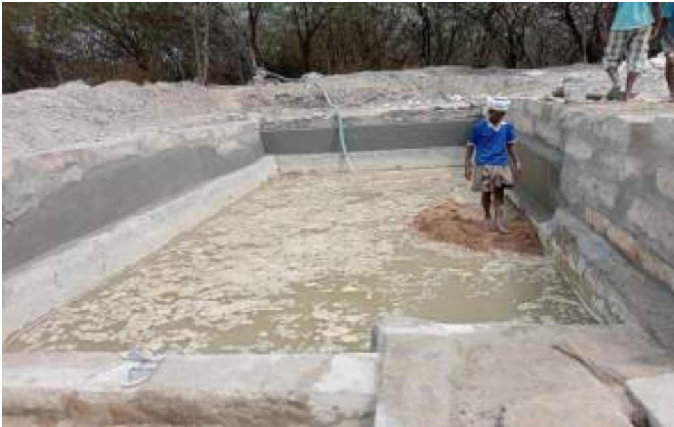
Spreading of sand - \frac{1}{2} feet throughout the Teertham base for better maintenance
