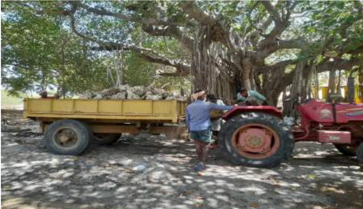
Construction materials unloaded on the way as the tractor cannot go further in the jungle as the area is wet land
