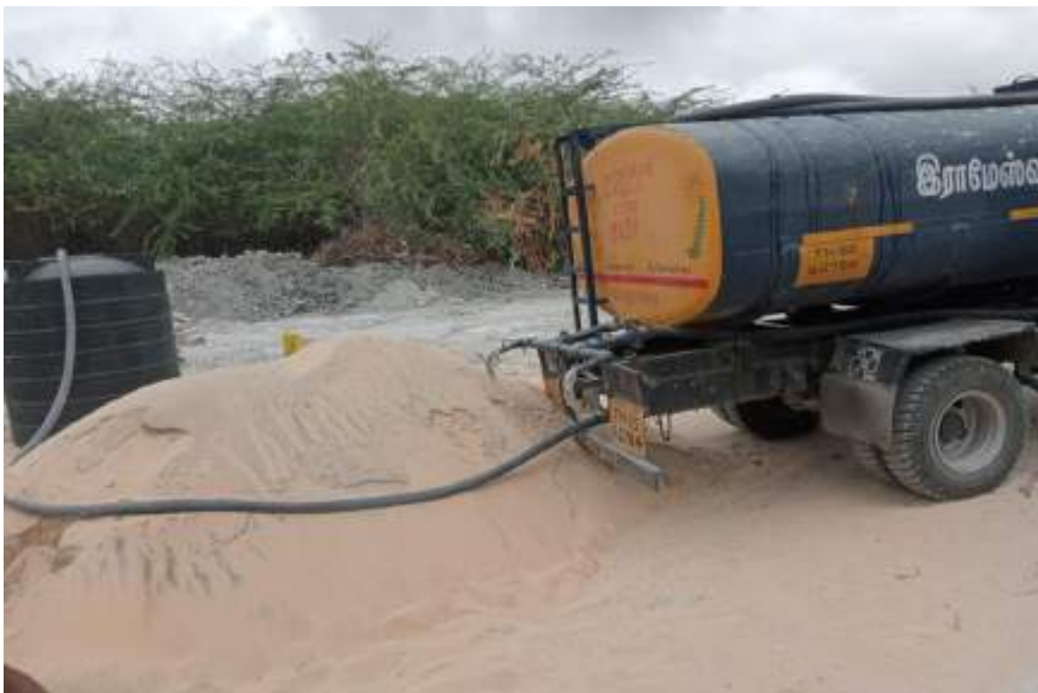
Good, fresh water is brought in a tanker for construction work as the local water is saline
