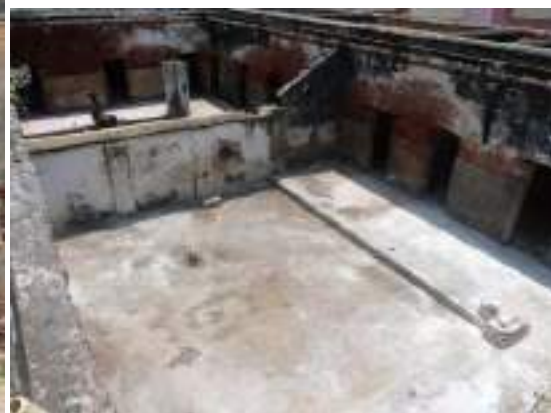
Damaged passage roof
