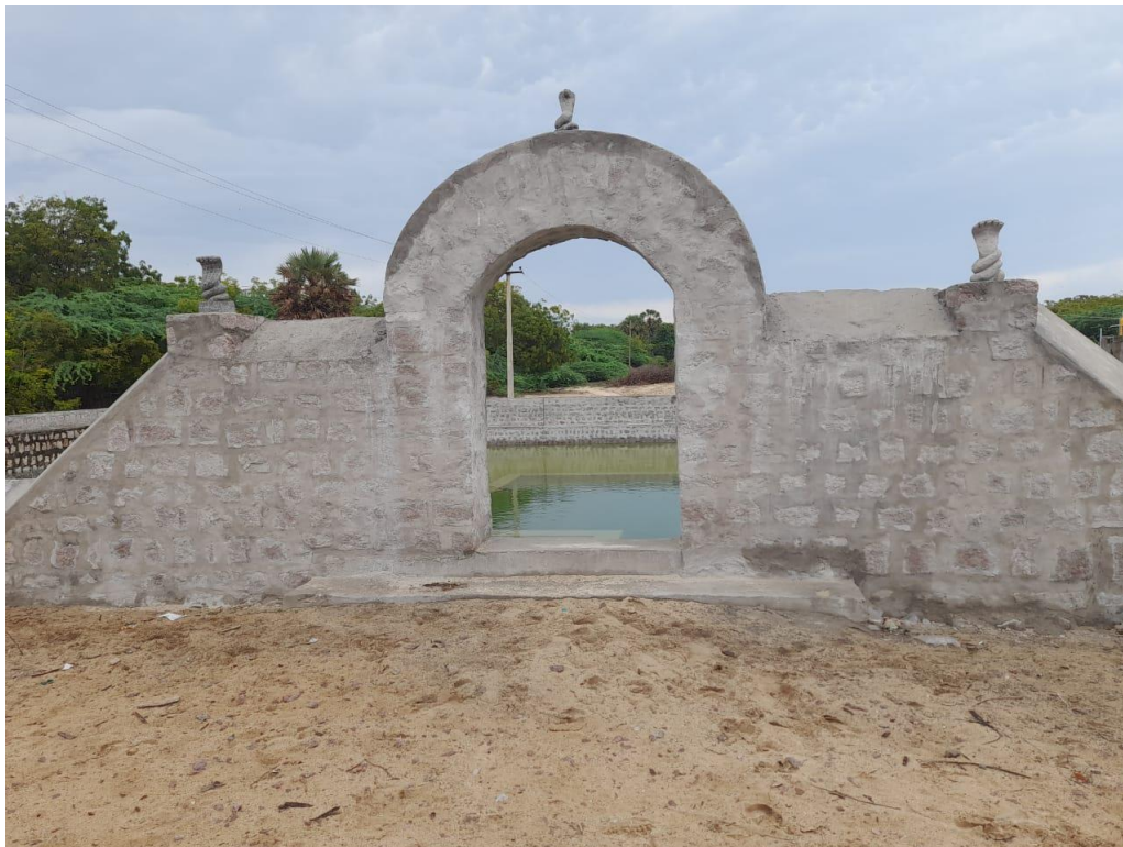
Construction of entry gate is in the final stages. Waiting for the door
