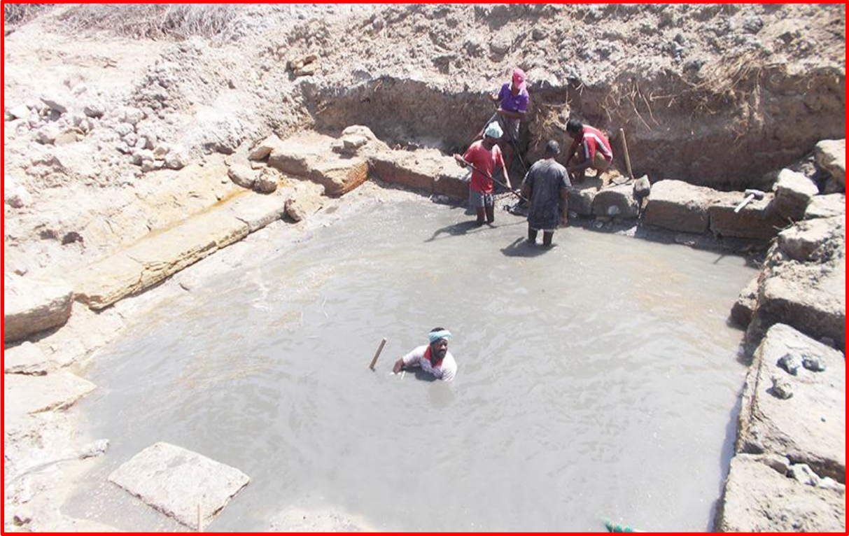
Worker de - silting manually and others busy in constructing the side wall
