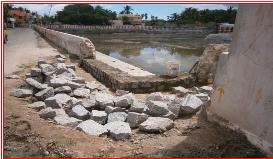
Teertham with dilapidated walls
