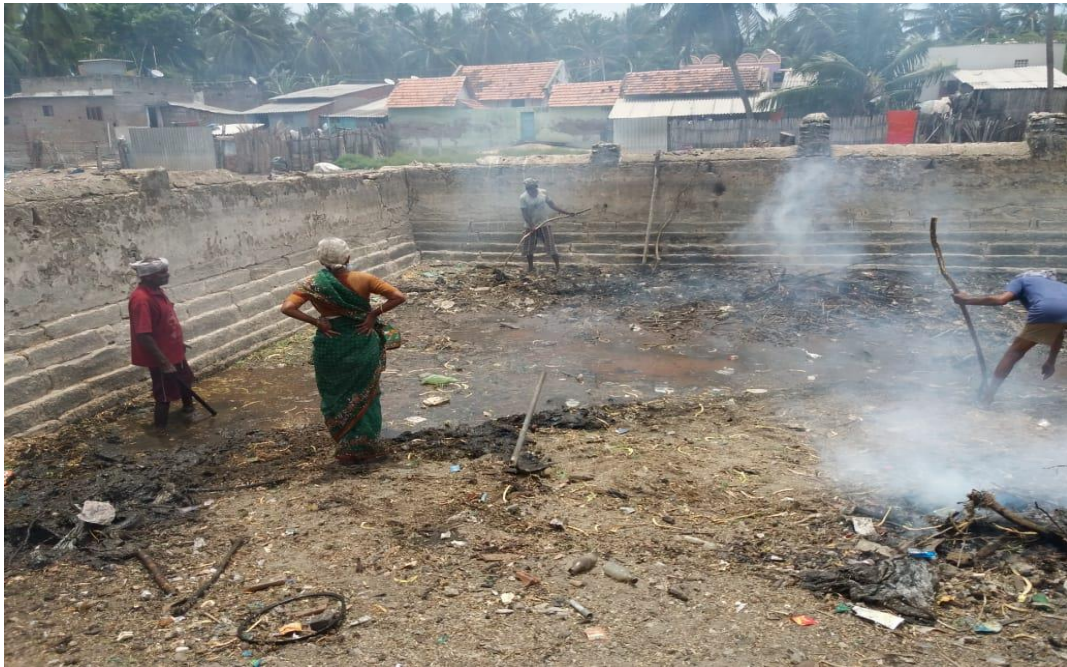
Inside structure of the dilapidated Parameswara water body
